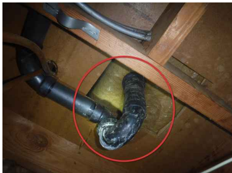
Leak under hall bathtub
