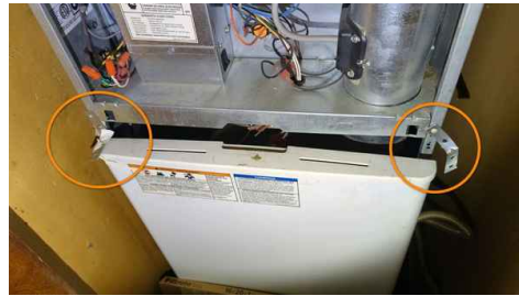
Brackets added because cover doesn't stay in place well
