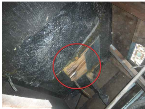
Water dripping down under primary bathroom shower
